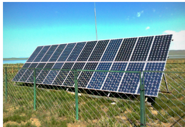
Figure 2 a: Solar array in Mongolia [8]
